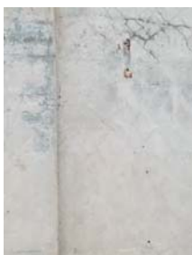
Peeling Paint And Anti Graffiti Coating - Tower Walls 3
