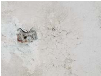
Damage Wall - Tower
