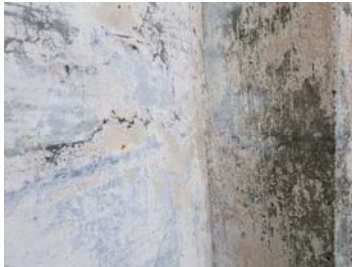
HMS-M17224-07A 3rd Story Coating at Column
