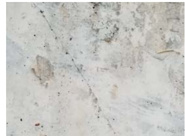
Peeling AGC and Paint
