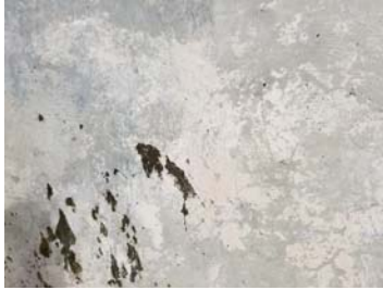
HMS-M17224-04A Deteriorating AGC and Paint
