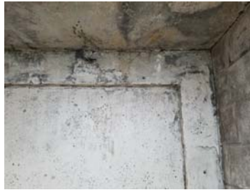
Damaged Paitn At Sealed Door to Tower
