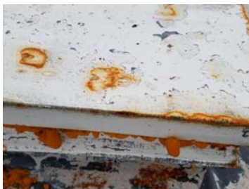
Peeling Paint - Tower Roof
