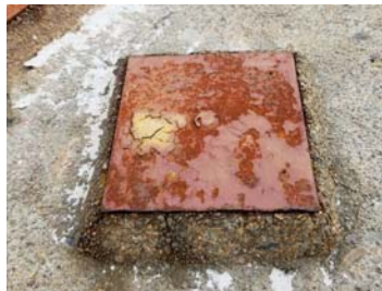
HMS-M17224-24A Paint on Brackets and Stands
