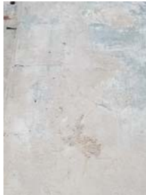
Peeling Paint - Tower Walls
