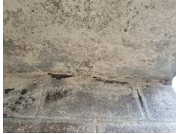
Peeling Paint at Entry Ceiling
