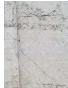
Peeling Paint And Anti Graffiti Coating - Tower Walls 2
