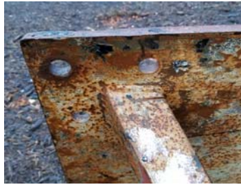
HMS-M17224-114A Mastic on Winch
