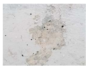
Peeling Paint And Anti Graffiti Coating - Tower Walls 5
