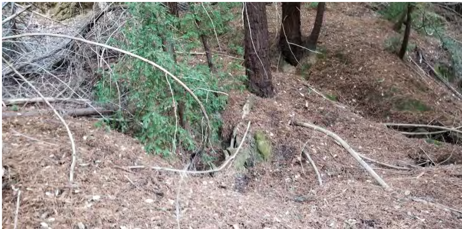
Photo 7: Two gullies at partially washed out watercourse crossing. The upper gully is from diverted stream flow coming down from MP8. The lower gully is from the watercourse.
