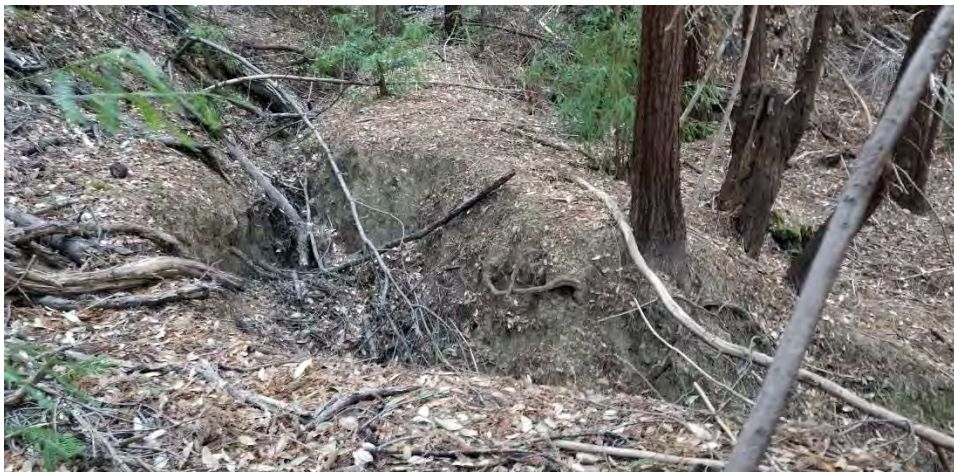
Photo 10: Looking up the road at the first gully. The second gully located in the opposite direction from how photo was taken is much larger.
