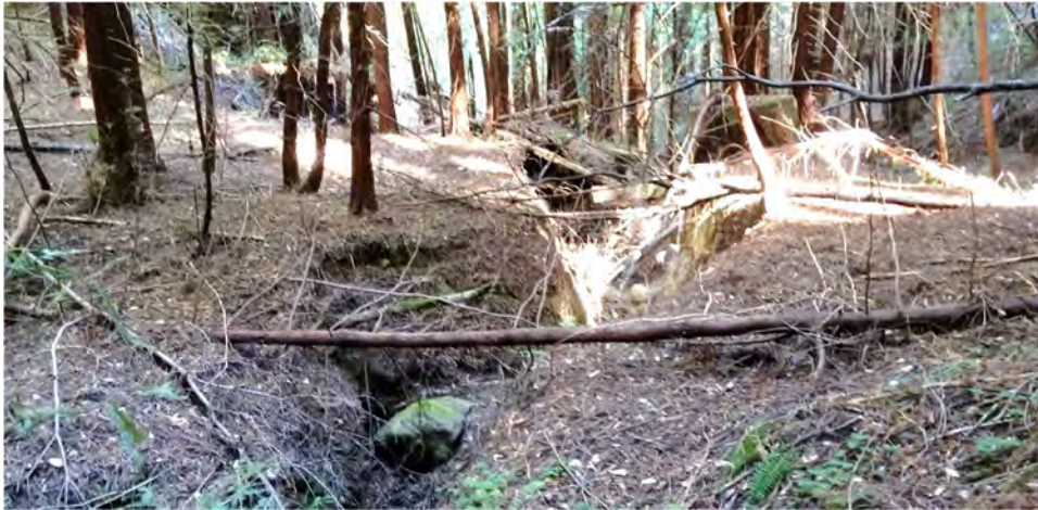
Photo 13: looking downstream at the partially washed out Humboldt crossing. Stream flow drains underneath a fallen stump just to the left of the eroded channel.
