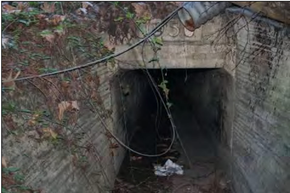
Figure A11: Culvert 1, west side, located at ravine, not visible all the way through.
