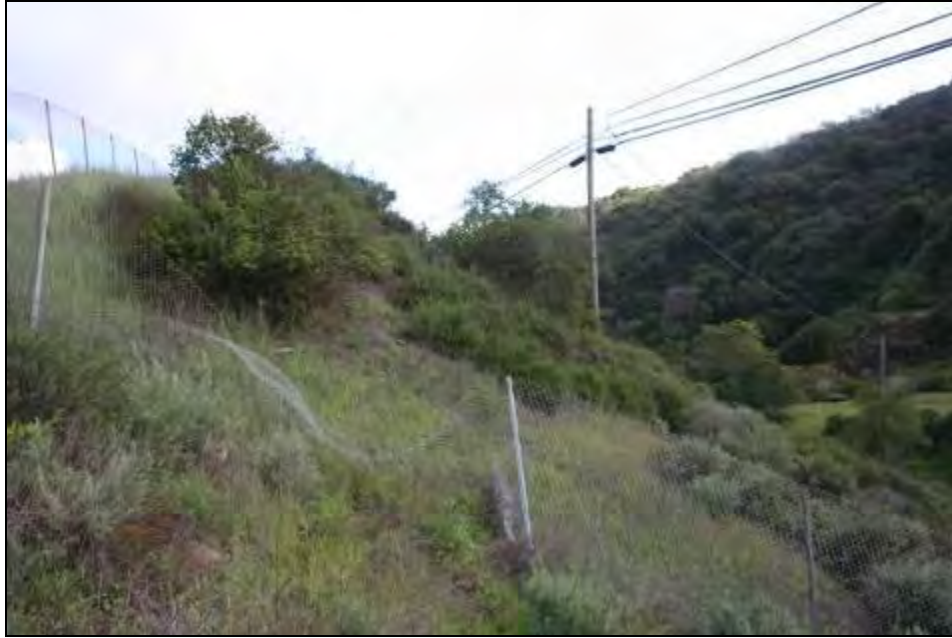
Figure A4: Fence down above Culvert 2 looking from highway down to Lexington County Park.
