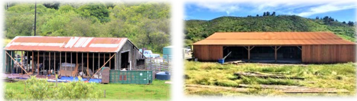
Figure-7: The wood frame barn (left) while under repair in May 2019 and post construction (right) in December 2019. The barn is located in the farmyard area near the main entrance to the Ranch off Higgins Canyon Road.
