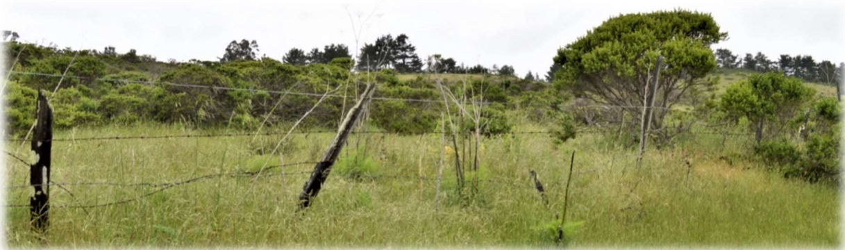
Figure-20: Old fence in poor condition with several loose/missing wires and broken wooden posts.
