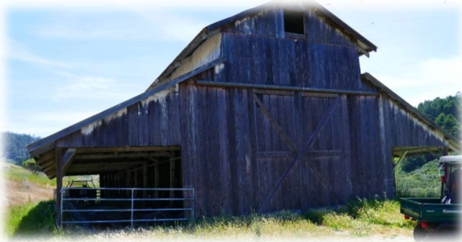
Figure-12: Old barn located along the southern end of the Hidden Valley grazing unit. The barn is in good structural condition and currently used by the grazing tenant to store hay and other ranch equipment.
