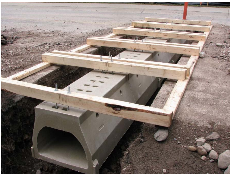
Herp (amphibian and reptile) crossing under construction - Waterton National Park, Alberta, Canada
