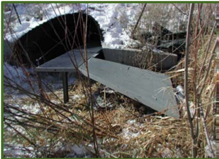
Figure 31: Example of raised catwalk inside culvert – Roscoe Steel and Culvert Co. and University of Montana’s “Critter Crossing”
